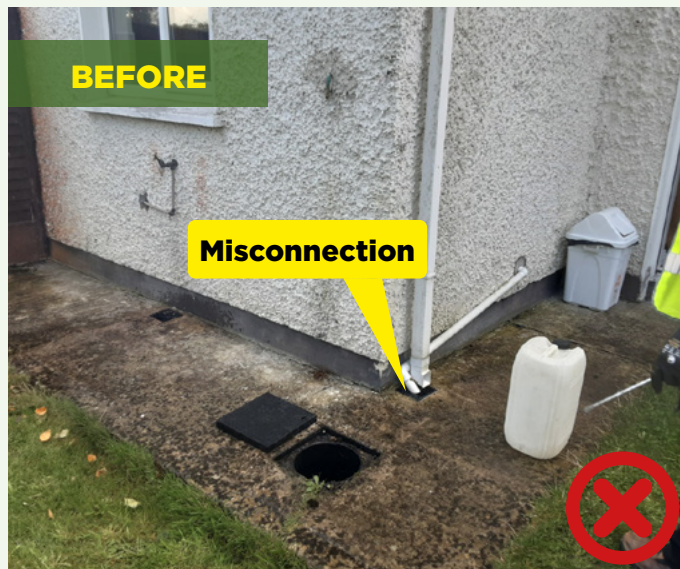
Typical domestic misconnection
