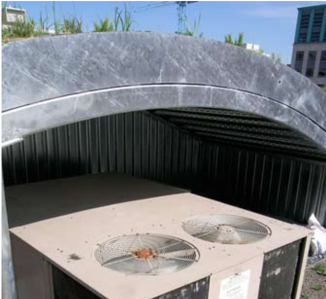
Figure 2.2 A Portion of the roof or 'wave' sits over air conditioning unit (courtesy D Saunders)
