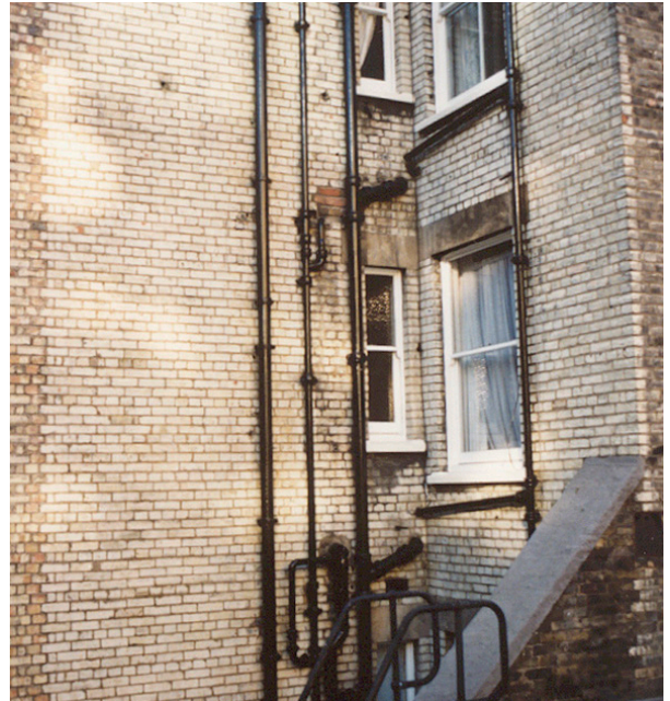
Figure 9: White walls require regular maintenance or their reflectance will deteriorate, as shown here
