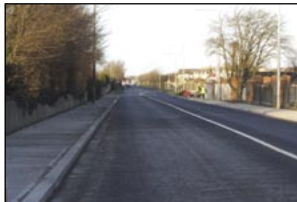
View along the improved section of the R120 Newcastle Rd. looking Northbound (towards Lucan Village)
