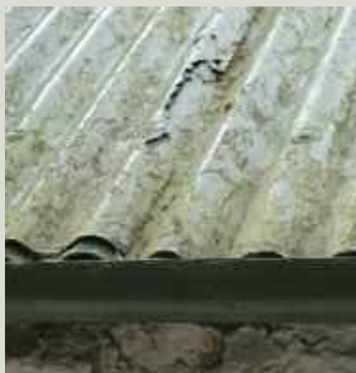
Crevice corrosion is frequently a problem with corrugated iron, particularly at the laps between corrugated sheets
