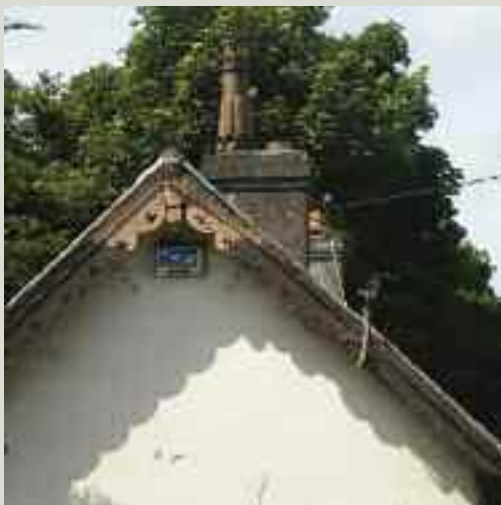
The poor condition of overhanging verges can lead to deterioration of the ends of the purlins as well as the loss of sections of decorative timber bargeboards
