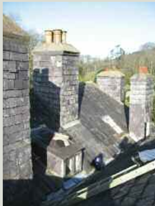
The change in colour of the slate on the chimneystack in the background indicates where a number of courses were removed and replaced. In areas of extreme weather exposure, vertically hung slating gives increased protection to the stacks
