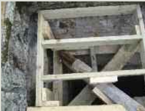
Additional support was added on the diagonal below the truss end, thus avoiding the need for new timber splice and steel connections or the local removal of the rotten timber truss end. The timber that had supported the gutter above had to be fully replaced
