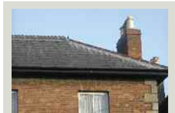
Incorrect bedding and detailing, with fat joints to the ridge and hip tiles, are visually very disruptive and inappropriate to a historic building
