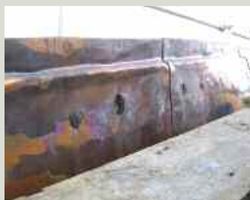
This copper parapet gutter lining has been lifted for inspection following water penetration problems. The bright salmon-coloured areas indicate that corrosion is occurring. Holes in the copper had been previously filled with a bitumen product in an earlier repair attempt which has exacerbated the problem, as bitumen corrodes copper
