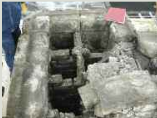
Many older flues have little more than half-brick fin walls called 'feathers' within the stack separating the flues from each other. These can be poorly tied in or even entirely missing as the result of chemical attack from soot, heat damage or over-vigorous cleaning with soot brushes
