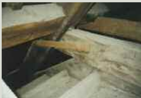
The extent of movement in this roof truss is serious, indicating not only the poor quality of the original detailing but also potentially serious movement in the main supporting walls below
