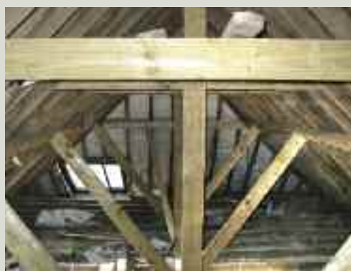
These rafters were originally undersized for their span and had deflected, causing slates to lift or slip, and thus allowing water to enter the roof space. To correct the problem, this additional support structure was added during roof repair works
