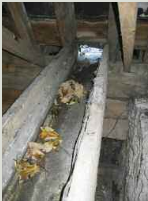
A lead-lined, secret gutter within the roof space used to carry rainwater from an internal roof to outfall at the eaves
