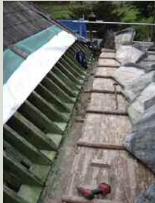
Slight lead corrosion can be seen on the exposed underside of the lifted lead sheeting on the right. The main problem here was a poorly detailed gutter. There was no need to change the regime of the flat roof, although good practice would include an underlay between the deal boards and the sheet lead
