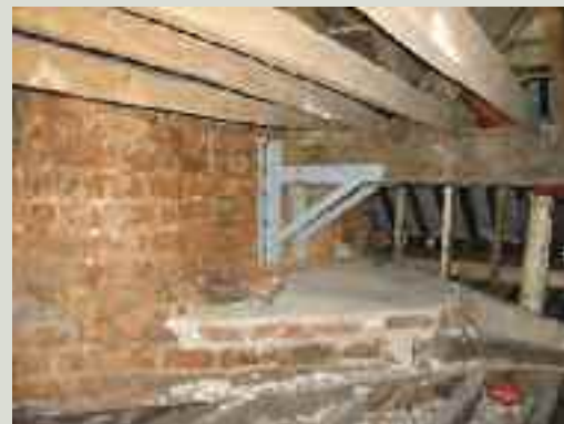
A new steel support bracket has been supplied to support this roof beam severely affected by wet rot at a chimney breast. The chimney flashings above, which had failed, were also repaired as part of these works
