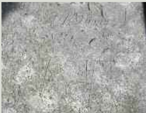
Lead sheet, while very durable, is soft. In this example, the lead sheeting has been etched with graffiti over centuries
