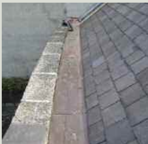
Parapet gutter re-lined in copper. The very shallow falls to this gutter precluded the use of lead
