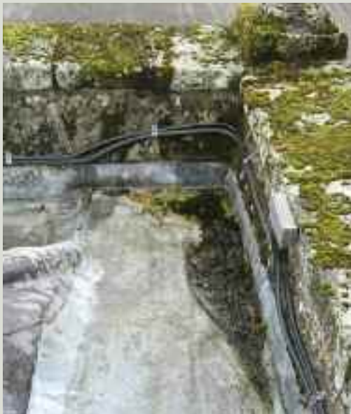
Ponding of water away from gutter outlets indicates a problem with the substrate timbers. In this case, a likely cause was poorly functioning flashings at the junction with the parapet wall
