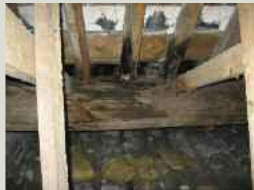
Evidence of wet rot damage to a roof beam and rafters under a tapered valley gutter. Only about ten per cent of the beam section was degraded, so no strengthening works were required to the beam. The rotted rafter ends, however, needed replacement
