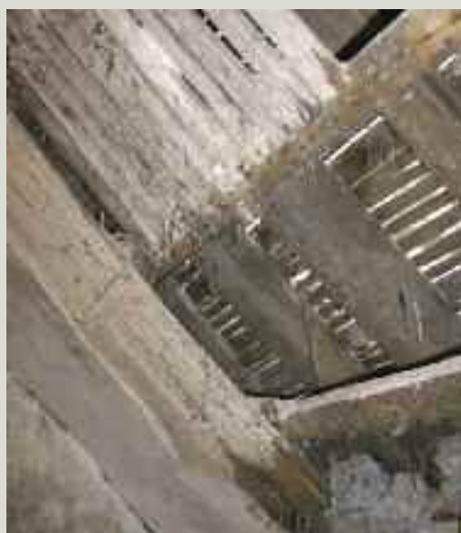
The recent discovery, within a later roof space of part of the former medieval friary in Ennis, of closely spaced riven laths fixed onto covered-over rafters substantiated the presence of an earlier structure within the historic fabric
