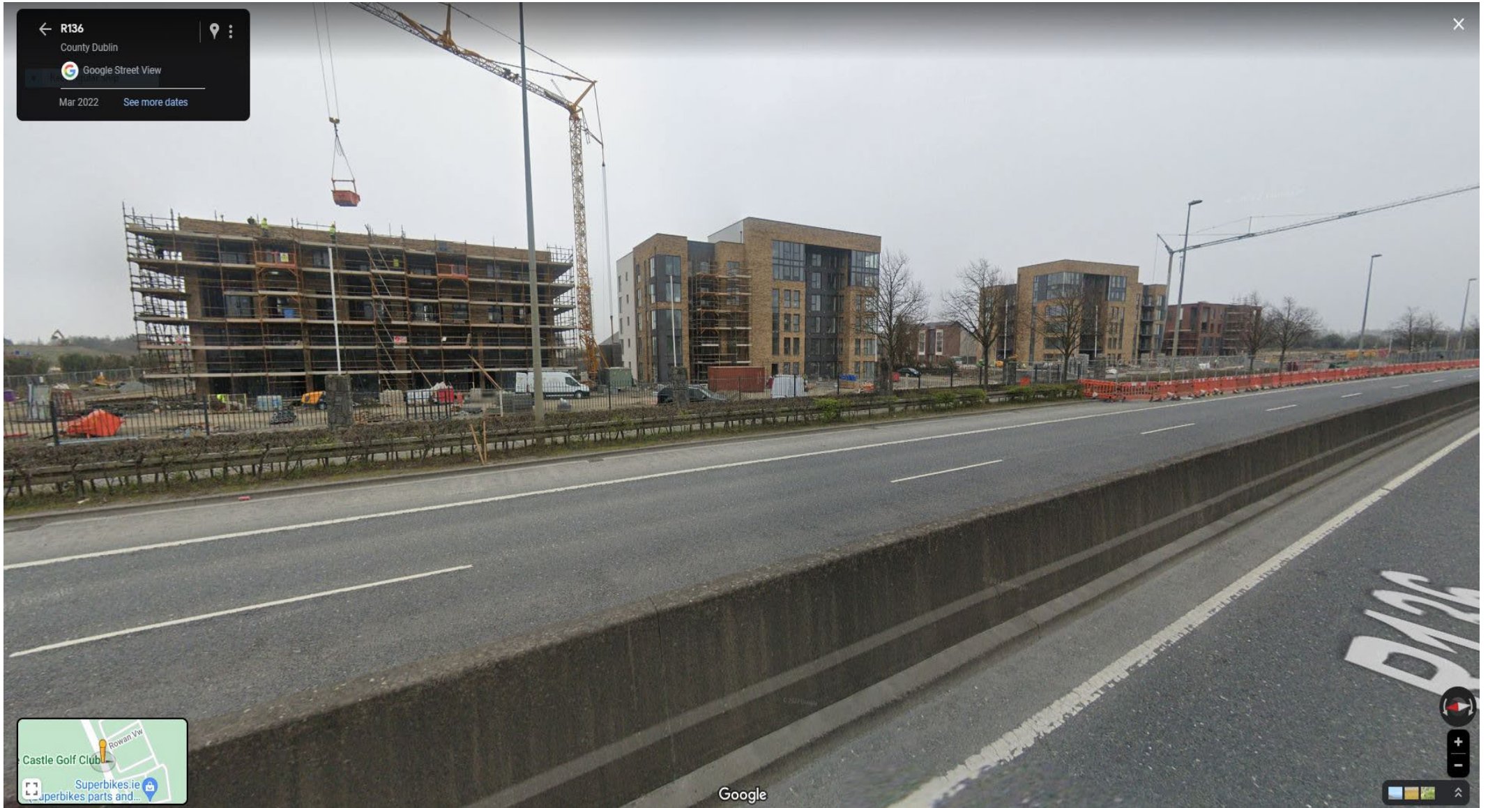
Google Street View of Development looking East from R136 (Image taken in May 2022 as per Google Maps)
