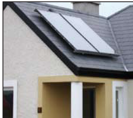
Example of solar panels on an extension.
