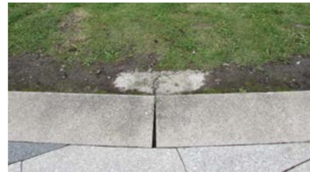
Image shows topsoil washout. The haunching is set near the top of kerb allowing for minimal topsoil to be placed, therefore prone to erosion over time.
