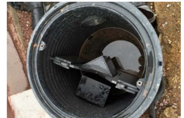
Images show a protected orifice plate within shallow chamber and weir made from recycled plastic planks.
