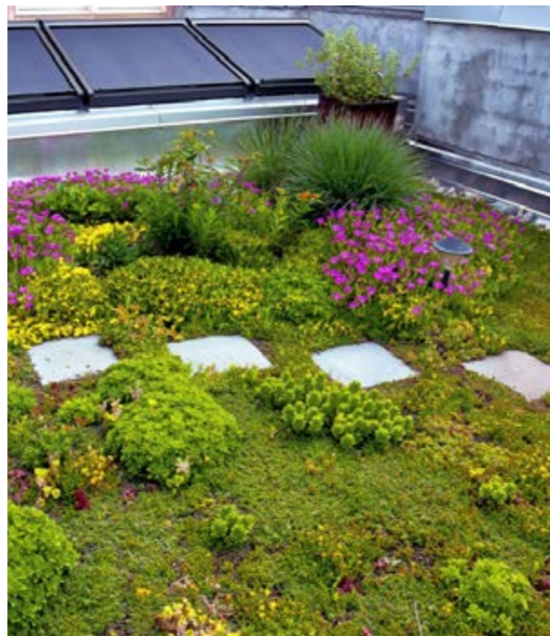
Green roofs can attenuate rainfall runoff where the outlet has a flow control (Blue roof).
