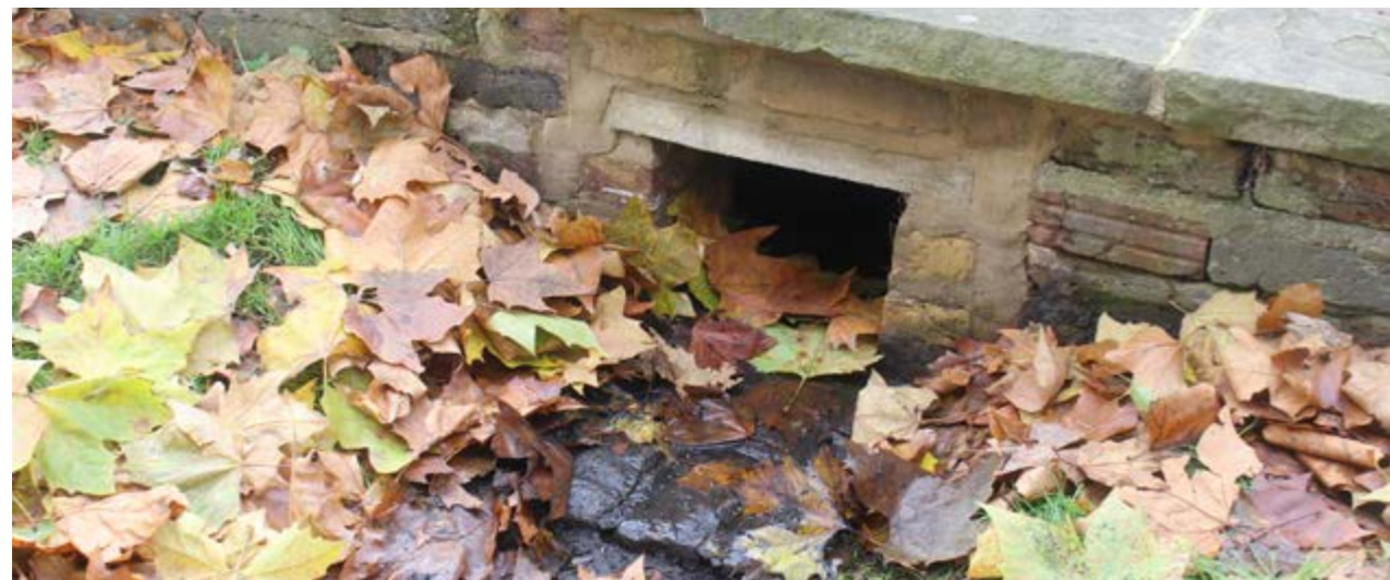
Polluted silts collecting from a busy road at an inlet apron allows for easy removal
