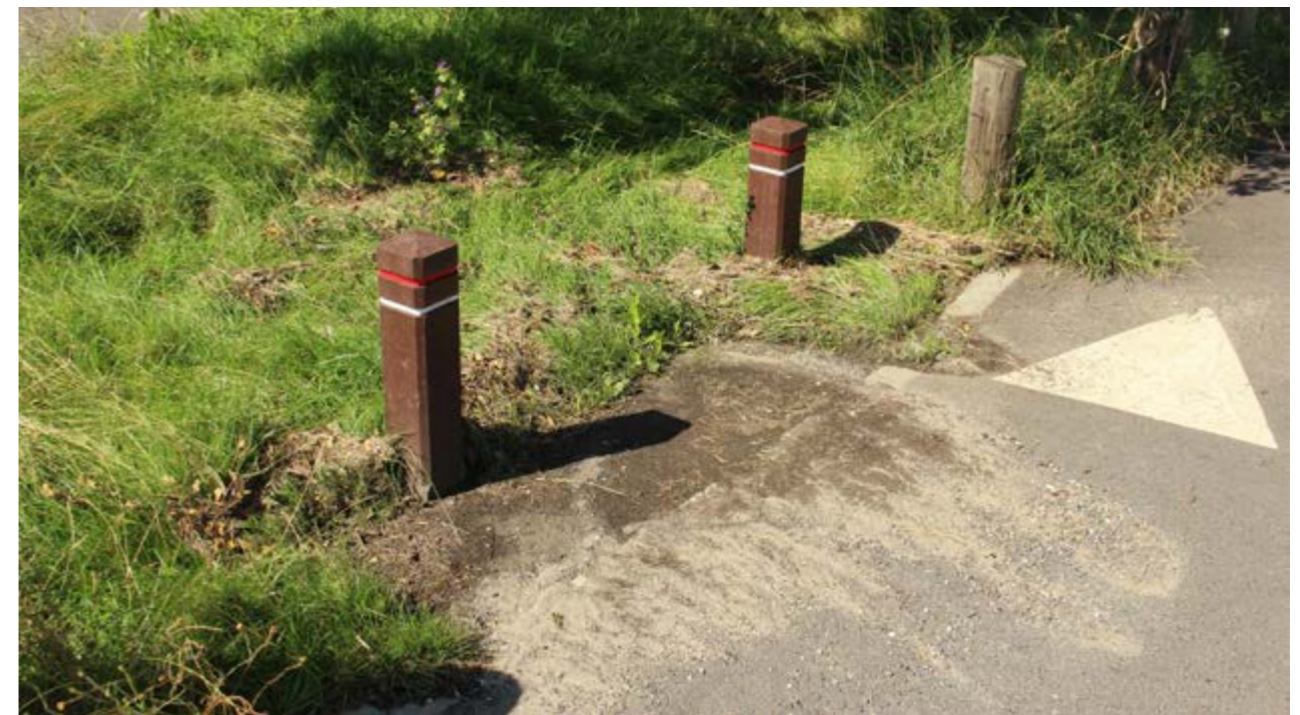
The gradual silt build-up at this kerb inlet into a swale was easily removed with a shovel.
