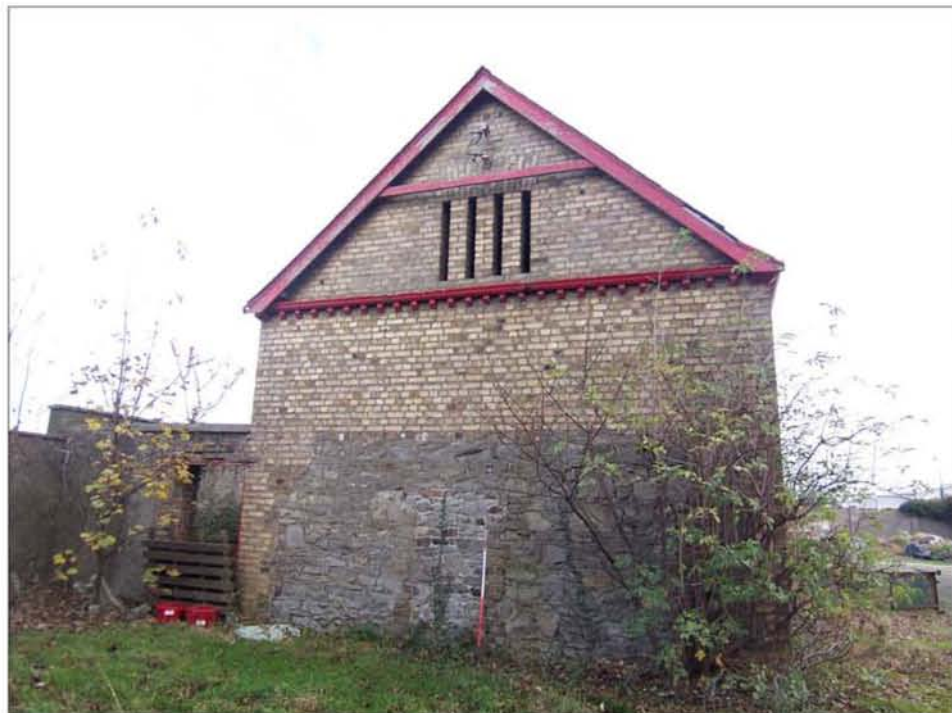
Plate 28 West gable of farm building (ID 3), showing masonry lower courses and blocked doorway
