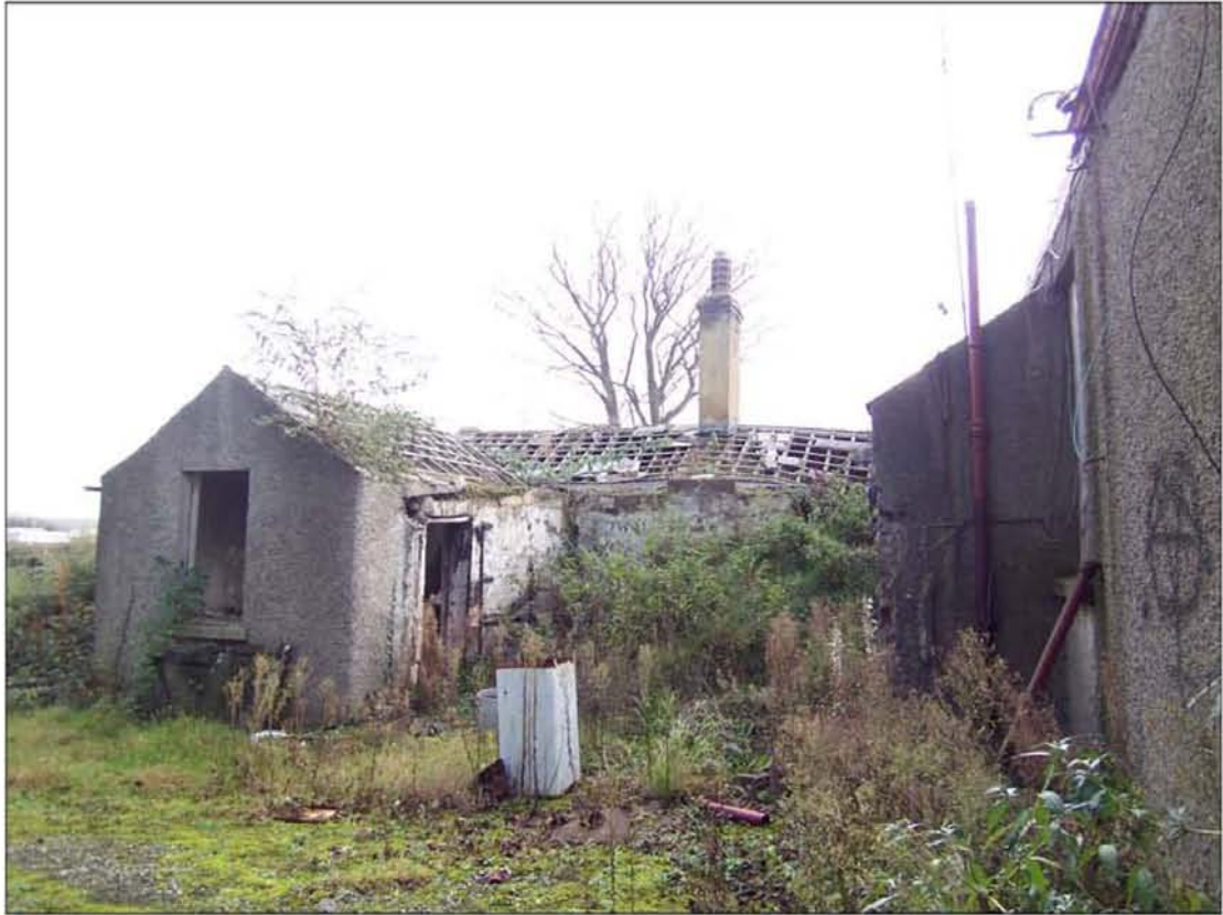
Plate 29 Later extensions to Newlands Villa (ID 2), showing extent of fire damage
