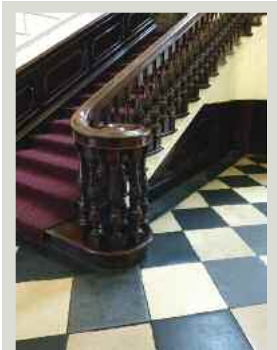
Solid stone floor: upgrading a stone-flagged floor such as this would inevitably result in an unacceptable level of damage or breakage of individual flagstones and should be avoided
