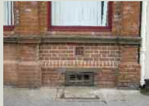
A floor vent to ventilate the ground floor was built into the wall between the cellar and ground floor windows as part of the original design
