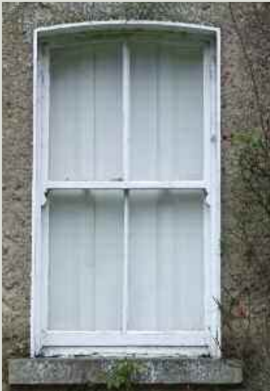
Working timber shutters: the interior of the shutter boxes could be lined and sealed to reduce air leakage. Any new linings should not prevent the shutters from folding back into the shutter box when not in use
