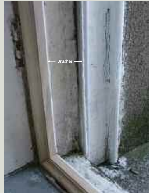
Draught-proofed window frame: brushes are visible on the staff and parting beads, both of which have had to be replaced in order to draught proof. For the brushes to work properly it is important that they are not painted over
