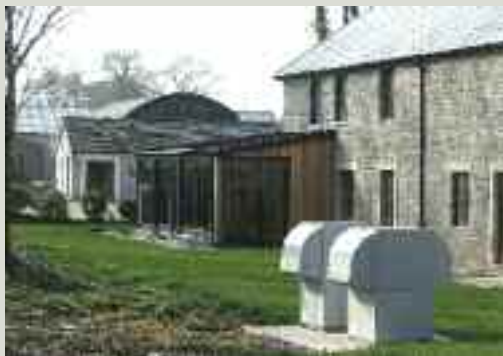
Air-to-water heat exchangers: a heating system provided to a converted stable building. The grey metal casing will be camouflaged by future planting
