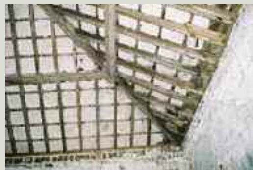
A roof with largely intact lime mortar parging applied to the underside of the slates. Parging has an insulation value in itself and helps to reduce air-blown water infiltration
