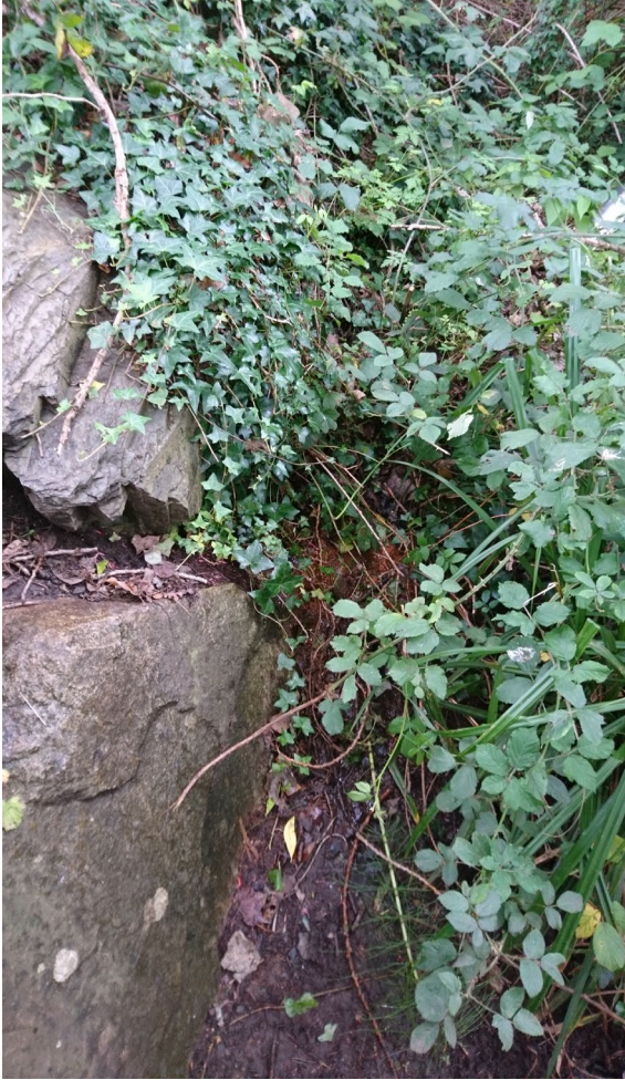
A 6: Seepage D05, hidden below vegetation
