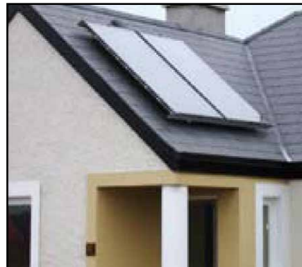
Example of solar panels on an extension.
